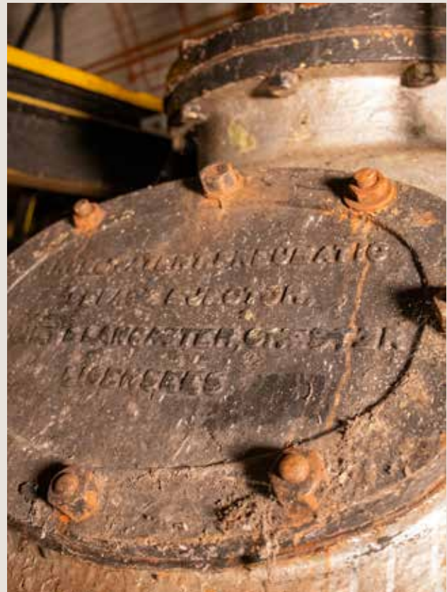
Original Victorian equipment
